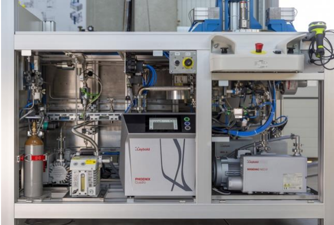
Leak test system for fittings: Implemented in this is a PHOENIX Quadro and a Leybold NEO D rotary vane pump
