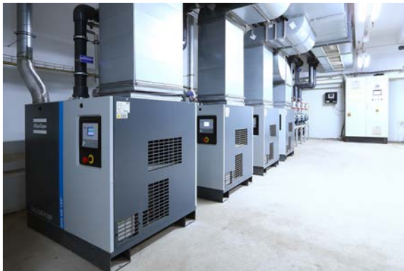
Central vacuum station 1 comprises four variable-speed screw vacuum pumps of the type GHS 585 VSD + and five boosters.
